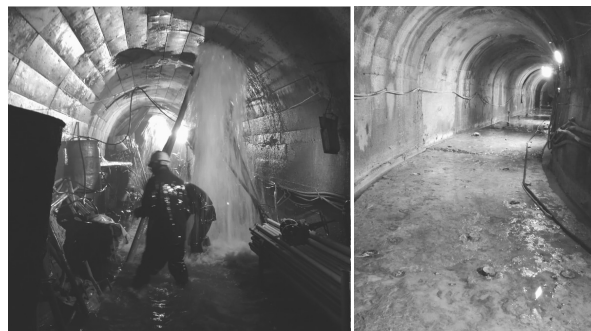
图 2 右岸 1340 m 灌浆廊道灌浆前后现场照片 Fig.2 The photographs of the 1340m grouting gallery on the right bank before and after grouting
