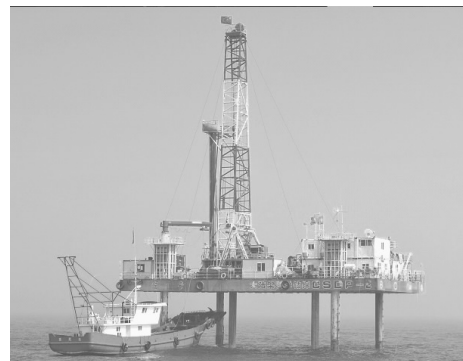
图 4 “探海 1 号”大陆架科学钻探平台施工现场图 Fig.4 Drilling site of “Tanhai No.1” continental shelf scientific drilling platform
