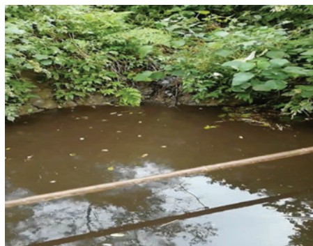
(c) ZK2-8未及时铺设土工布致油污污染水体
