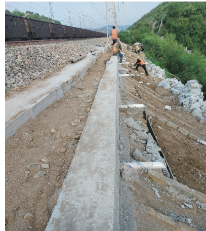
图 2 K319+200~380 下行侧路基下沉及注浆挡墙施工照 Fig.2 Construction photos of roadbed sink, grouting and retaining wall in the K319+200~380 downlink side
