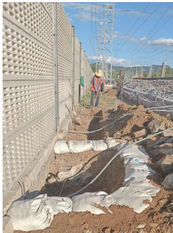
图 1 K319+200~380 上行侧路基下沉及注浆挡墙施工照 Fig.1 Construction photos of roadbed sink, grouting and retaining wall in the K319+200~380 uplink side
