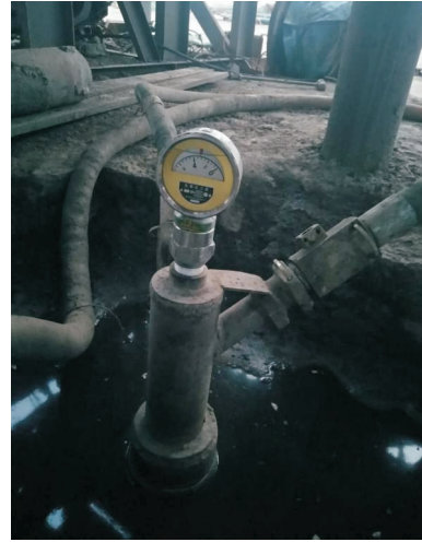
图5 传统钻孔压水试验孔口装置工作现场 Fig.5 Drilling field of conventional wellhead device for water injection test
