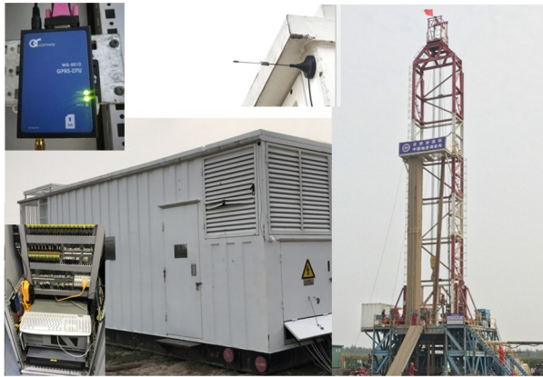
图 9 雄安新区地热井钻探现场数据采集系统 Fig.9 Data acquisition system for drilling at site of Xiongan geothermal well
