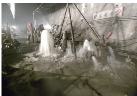
图 7 现场分流减压孔钻孔 Fig.7 Drilling of diversion holes for pressure relief
